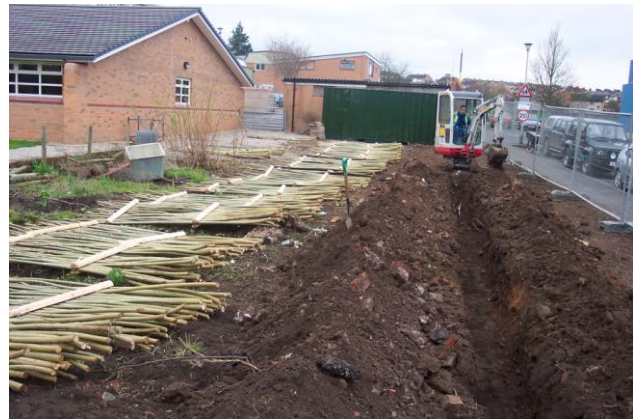
Willow panels laid out ready to plant once the trench is completed.
