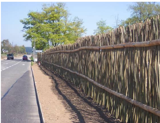
The Green Barrier in living Willow after completion. New growth will appear in spring.
