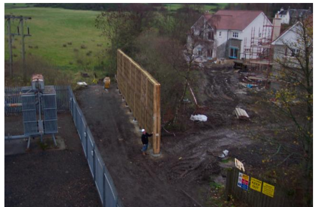
The Barrier screens the sub-station from the new houses close by. Climbing plants will be planted next to the Barrier to further enhance the appearance.
