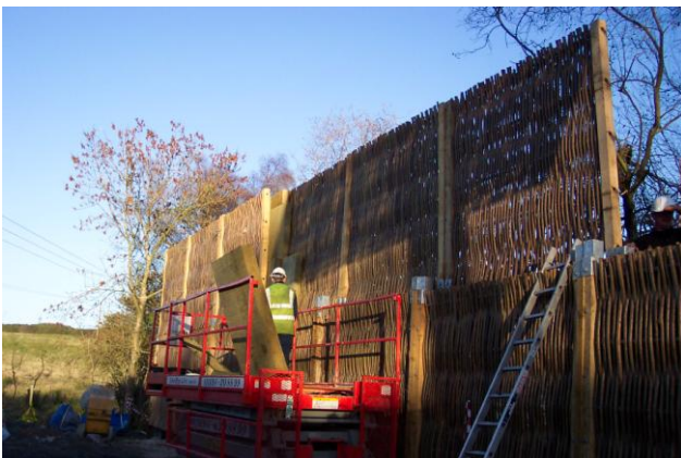
The RockDelta core being put in place between the Willow panels. The core will absorb much of the noise emitted from the sub-station.
