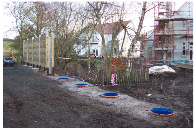
The base of the Green Barrier is concreted into place, giving stability.
